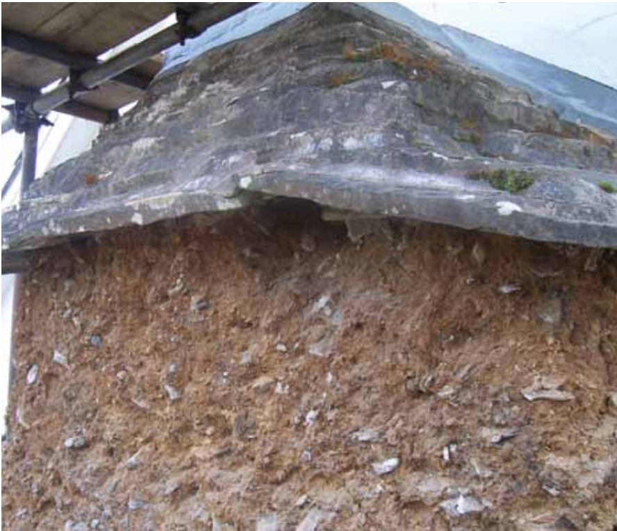
ABOVE: The overhang of this roof has kept the cob dry and stable. BELOW: Slates on and Watertight!
