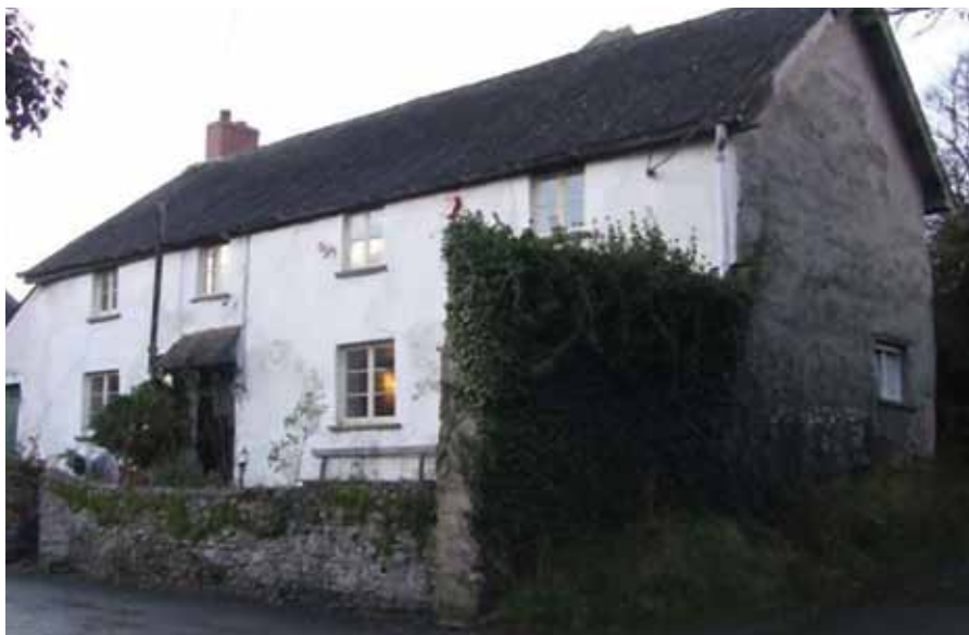
ABOVE: Before work begins removing existing roof and replacing with thatch. BELOW: New thatch has replaced old roof.
