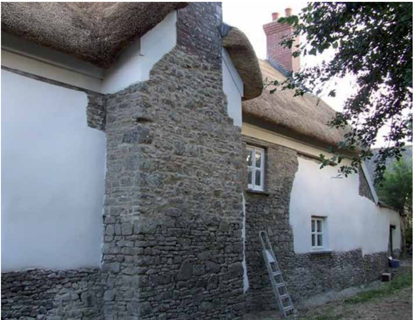
BELOW: Walls have been rebuilt and together with the stack are in the process of being repointed with lime mortar.
