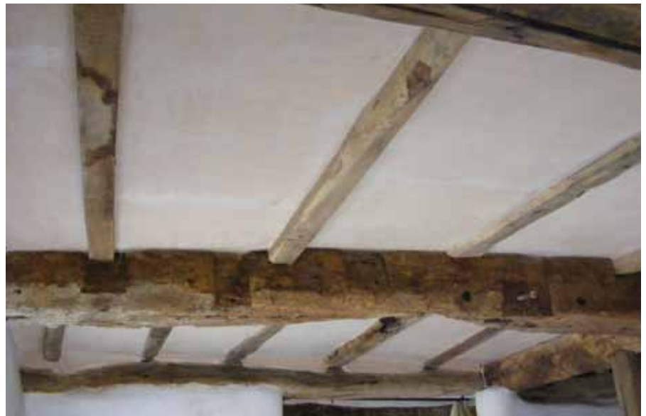
ABOVE: Ceiling restored, orange foam filler banished. BELOW: New staircase in place- walls re-rendered with lime mortar.
