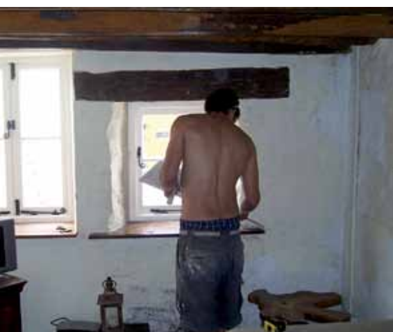
ABOVE: Note mildew on wall-stonework has been painted with modern paint.
