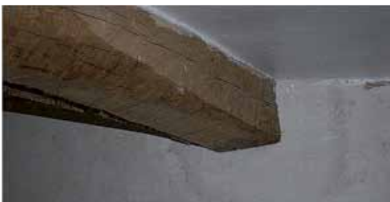
ABOVE: Beams may need replacing.
